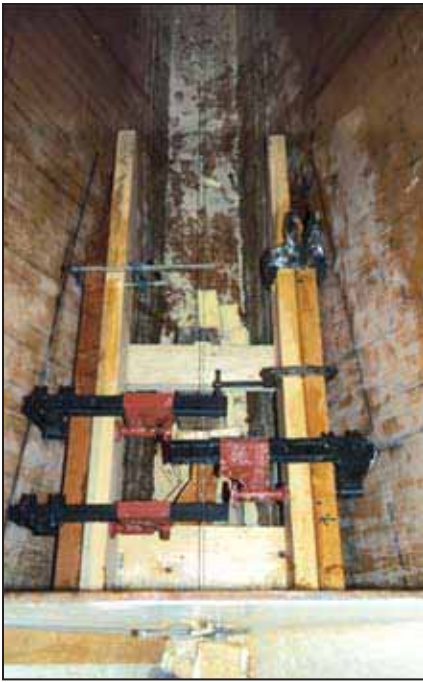
Engine beds glued together and clamped in position while the epoxy putty sets.
