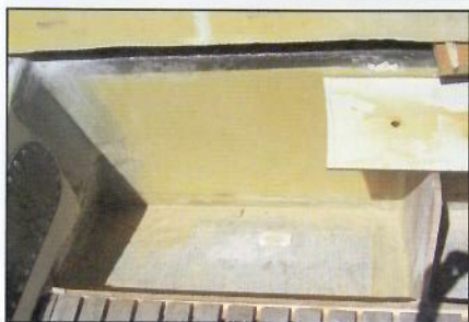
Lockers under construction. (top) The vacuum bagged panels have been taped to the existing cabin structure and some fairing compound has been applied to the seam. (bottom) New locker panels and partitions fiberglassed in place.
